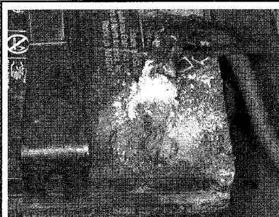
Fig. 91 Ignoring a battery (and corrosion) to this extent is asking for it to fail
